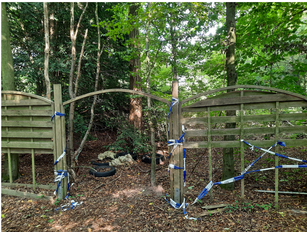
Figure 4. Gaps in the perimeter fencing of JHQ Rheindahlen used for unauthorised access.
