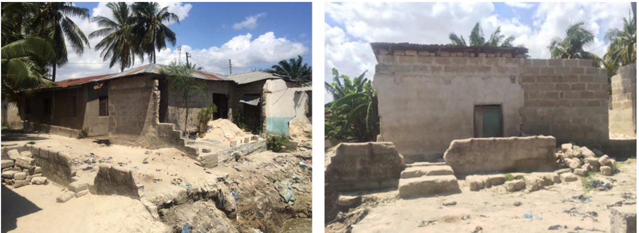
Figure 10. Damaged Swahili houses in Tandale by Ng'ombe River. Source: Courtesy of Beatrice Mahagama and Leticia George.
