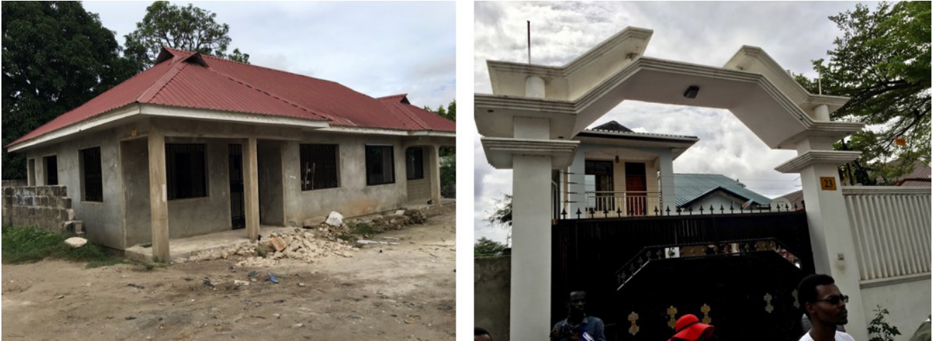
Figure 9. Renovation (left) and conversion of a Swahili house into higher-income, single-family homes (right).
