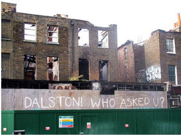
Figure 1. Key moment during the Dalston Lane controversy: Demolition of historically significant examples of early 19th century Georgian terraces on Dalston Lane after years of neglect and fire damage, 2007. Source: OPEN Dalston (2007b).
